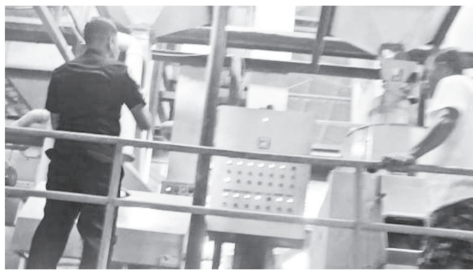
Conducted Fire Safety Inspection to all Industrial Occupancy in relation to the BFP Year Round Fire Safety Awareness Program dated 25 October 2018.
