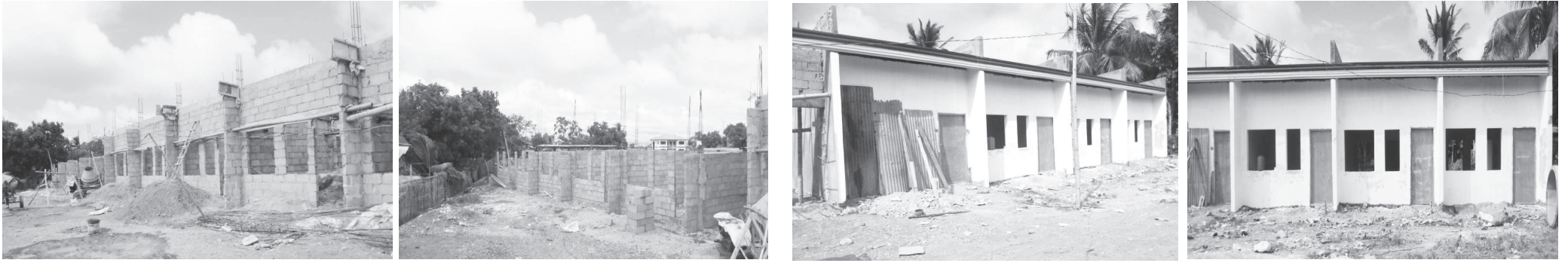
ON GOING CONSTRUCTION OF 24 ROW HOUSES, LOCATED AT MINA EAST, MINA, ILOILO
